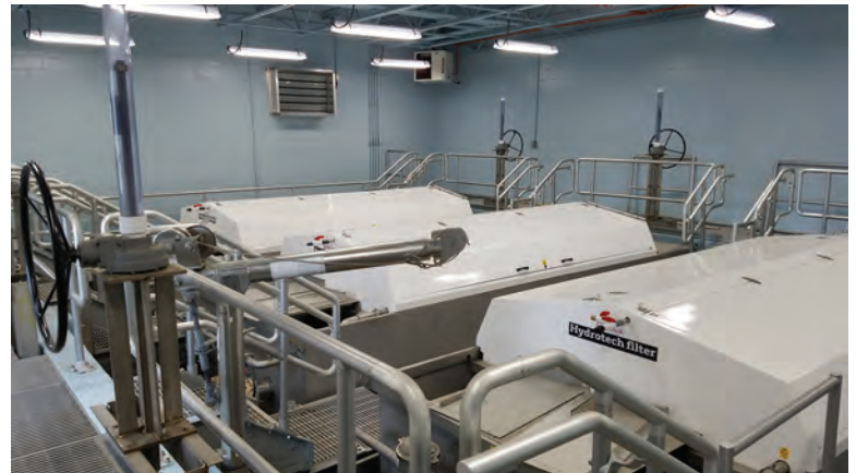
New disc filters (Veolia Water) have reduced power use at the Crown Point plant, saving the city about $70,000 a year.
