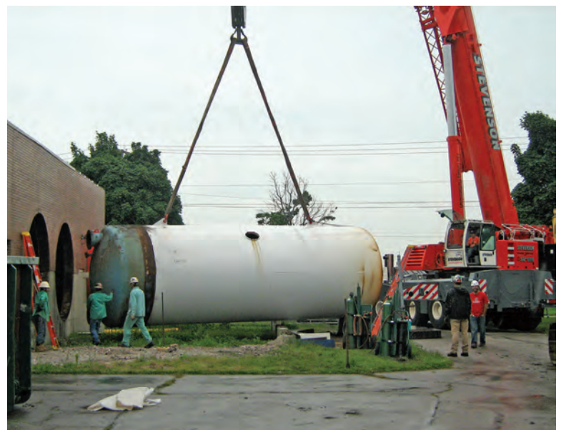
One of five pressure filters is removed from the Crown Point plant to make room for the new disc filters.
