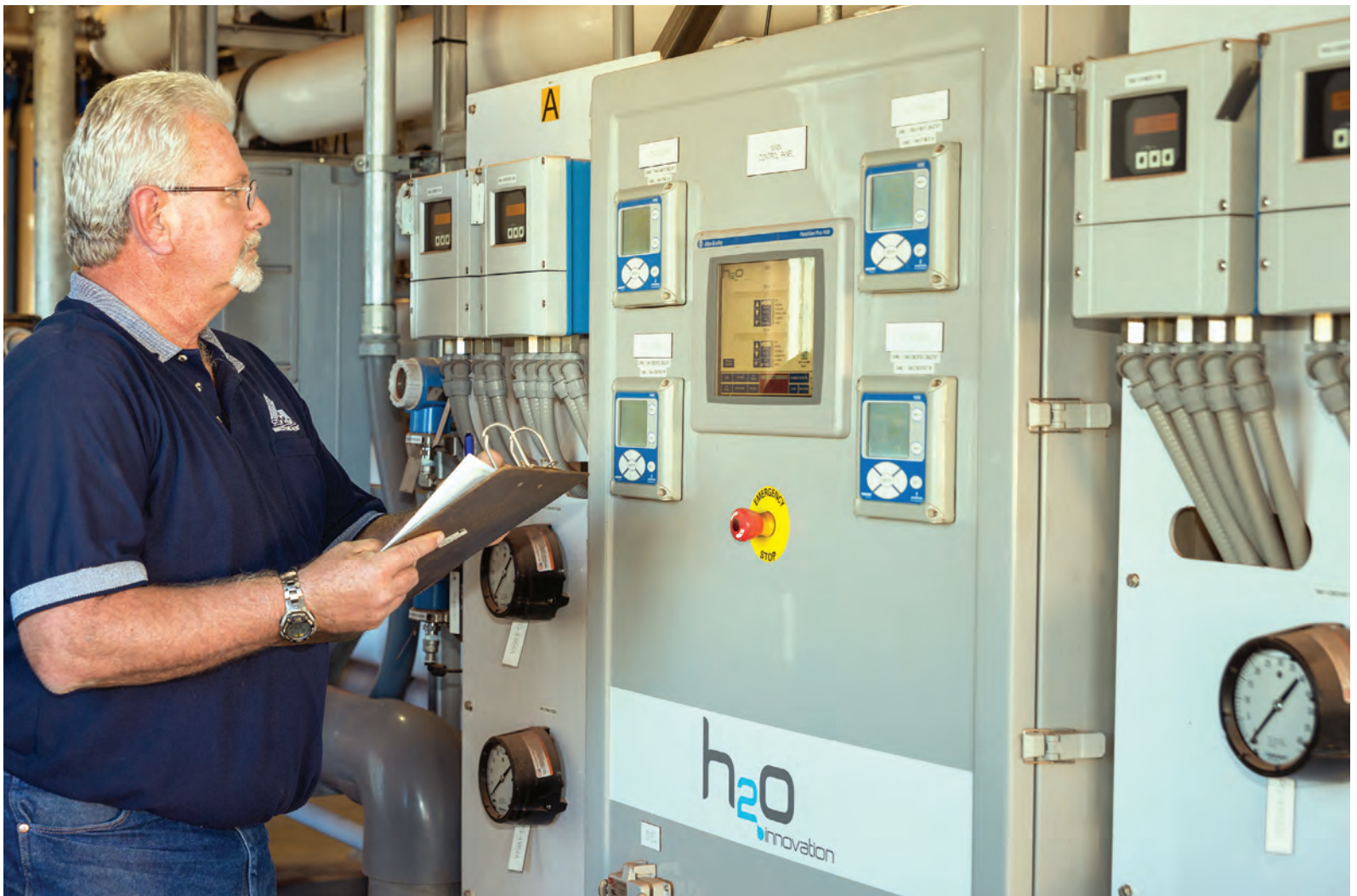
Garry Houston records process numbers on the plant’s third-stage concentrator (H2O Innovation).
