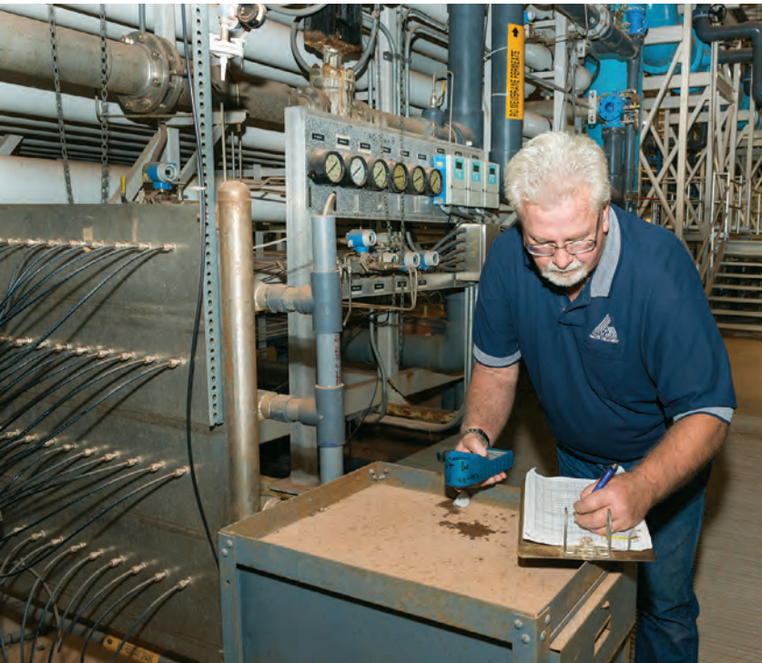
Houston takes sample readings at the reverse osmosis trains (Advanced Environmental Water Technologies).
