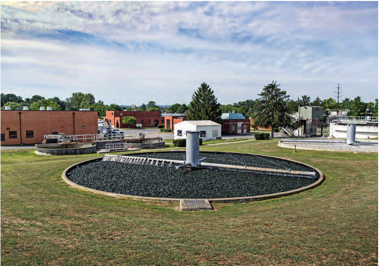
The 2 mgd (design) Mechanicsburg Wastewater Treatment Plant serves a population of about 14,000.
