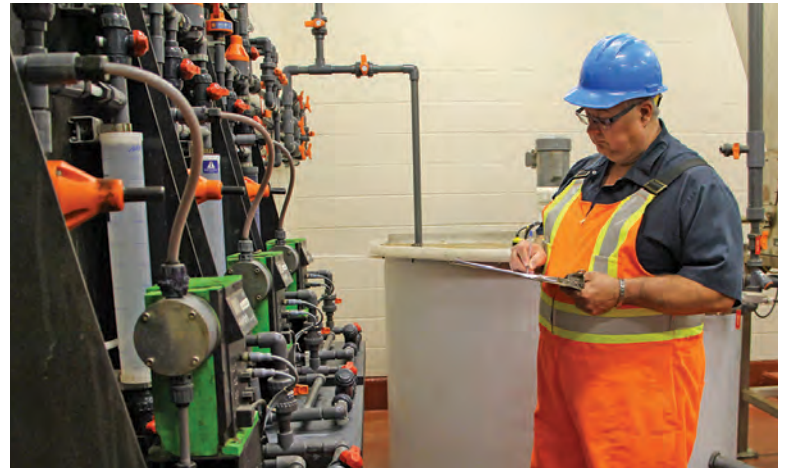
Operators including Norman Parachoniak had a hand in designing the new Queen Street Water Treatment Plant.
