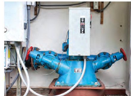
LEFT: Jim Jans (left), manager of the Corbett Water District, with David Jacob, owner of Hydra Engineering and designer of the district's hydro-turbine. BELOW: A jet on either side of the hydroturbine feeds water from an 8-inch supply pipe. The electrical box with disconnect lever is above the unit.
