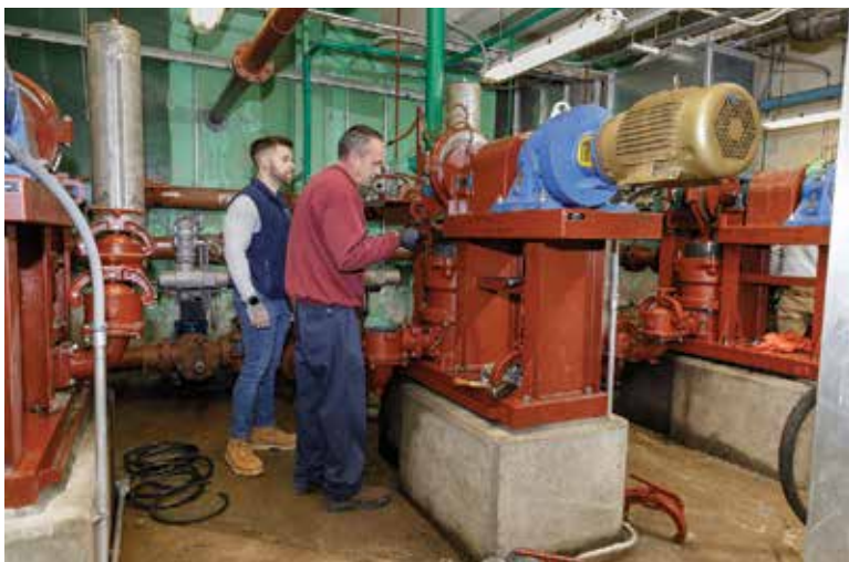
David Milano and Mark Carusillo install new packing in the primary sludge pumps.
