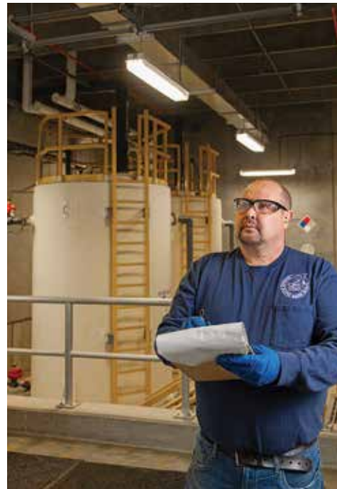
Rod Scott checks inventory levels, inspecting chemical feeders in the bulk container room, equipped with Pulsafeeder pumps.
