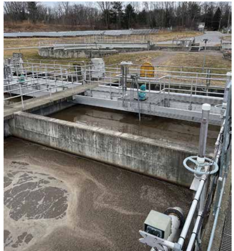
An anoxic zone for biological phosphorus removal was added to the treatment stream. It uses low-power mixers (INVENT) to keep the solids suspended without adding air.
