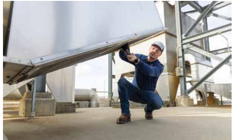
Ian Cassidy cleans an aerator screen to remove debris and maintain proper airflow atop the pretreatment building (Siemens, now Evoqua Water Technologies).
