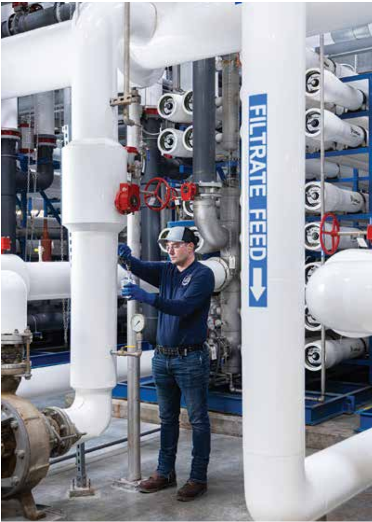
Ian Cassidy takes a sample at the influent to the RO membranes (Veolia) to confirm there is no chlorine residual.
