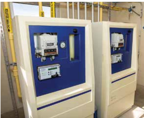
The water treatment plant draws from 51 wells. Chlorine is monitored by De Nora CAPTROL controller stations.
