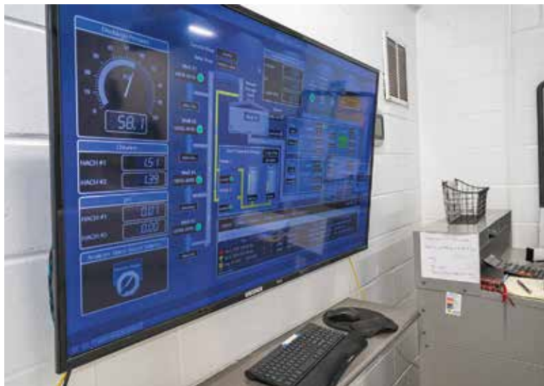
The SCADA screen at the University of Central Florida Drinking Water Plant.
