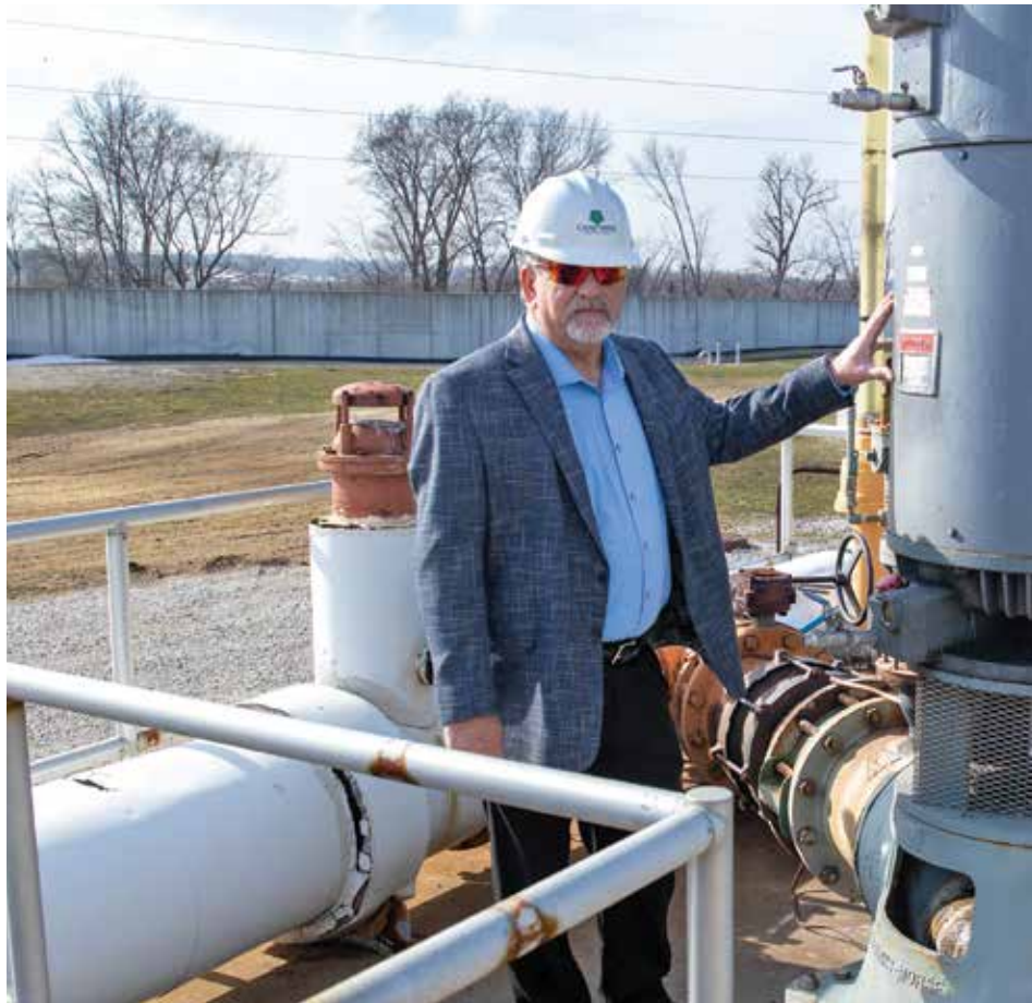
Roy Hesemann, Cedar Rapids utilities director, oversees two water treatment plants with a combined 60 mgd capacity (effluent recycle pump from Pentair Fairbanks Nijhuis).
