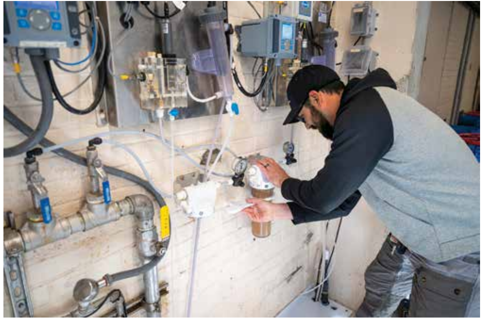
The university water plant includes extensive automated monitoring and control. Riley Baird, utilities specialist, is shown in the pump room (Hach monitoring equipment).
