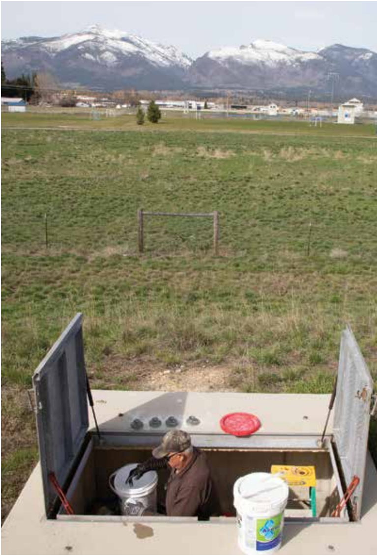
One of Steve Mosbrucker's many jobs is adding chlorine tablets (Norweco and Jet) to the system. This part of the treatment plant was scheduled for an update last summer.
