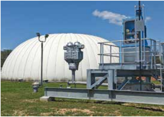
Digesters were upgraded and new mixers added when the Western Virginia Water Authority began converting its biogas to renewable natural gas.
