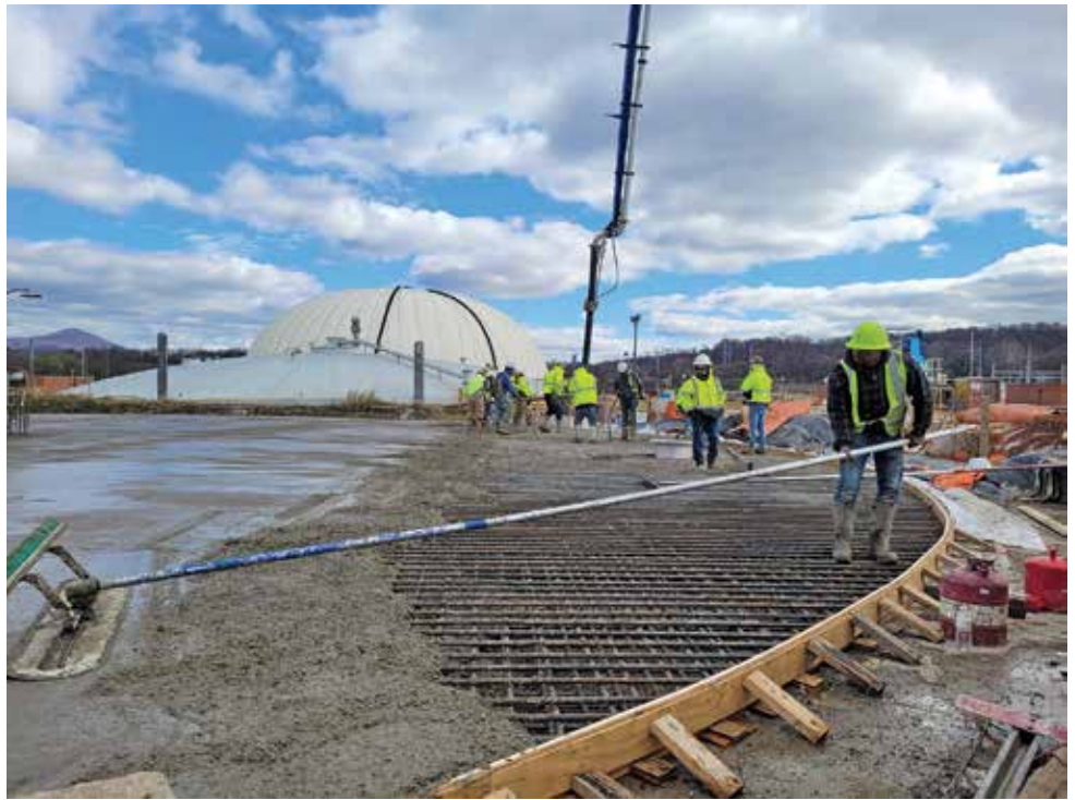
Workers spread concrete for a new digester at the Roanoke Regional Water Pollution Control Plant.
