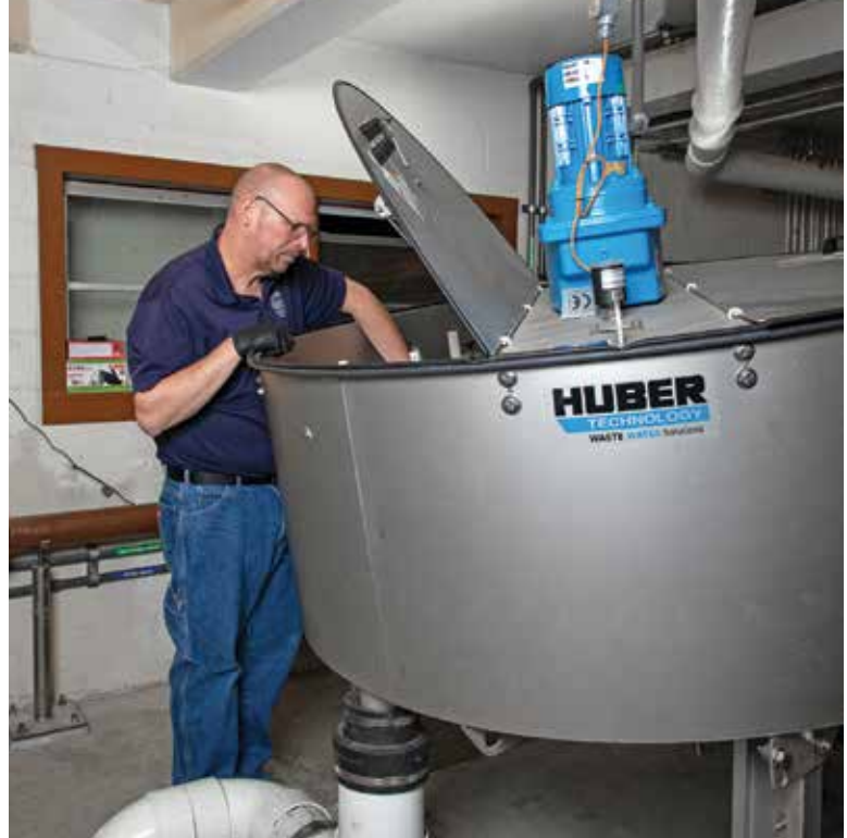
Todd Gianotti monitors the process on S-DISC sludge thickener (HUBER Technology).
