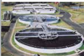
Spiraflo clarifier from Lakeside
