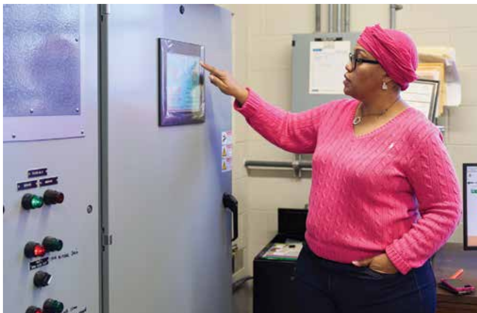
Oberton, shown checking water tower levels using a SCADA panel (Shorite Controls), emphasizes effective communication in dealing with team members.
