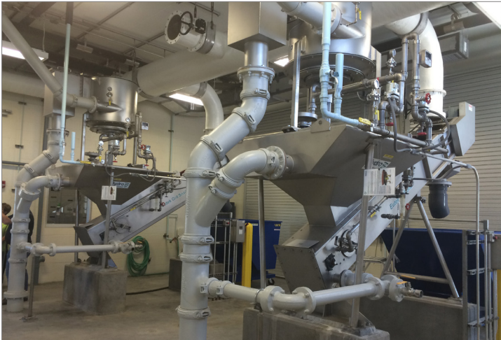
Grand Island’s SlurryCup / Grit Snail Washing & Dewatering Systems
